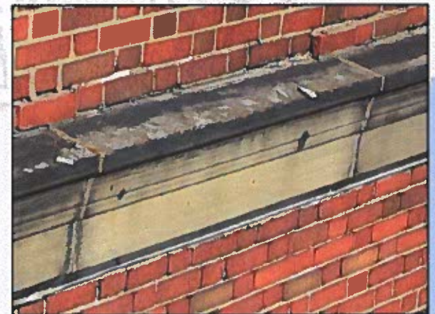
A loose stone cornice attached by metal fasteners indicate that its fasteners have failed.
