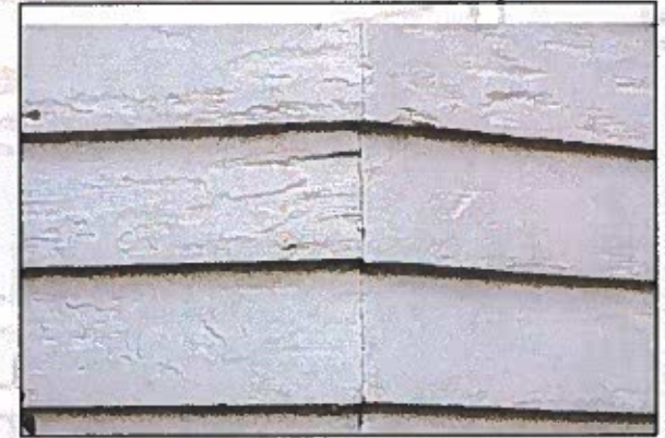
Improper preparation before applying paint results in a poor finish.
