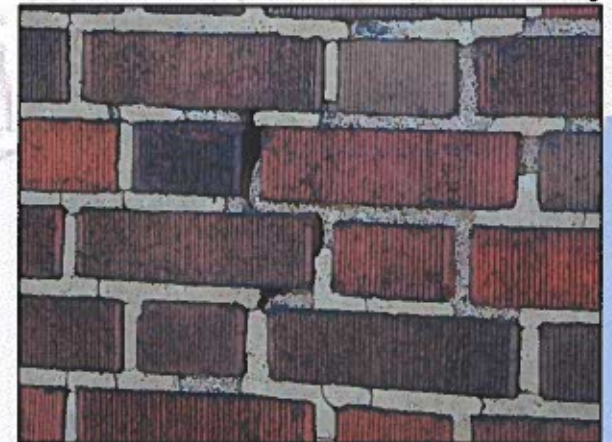
Previous poor repointing. Repointing mortar is falling out of joint due to improper execution.
