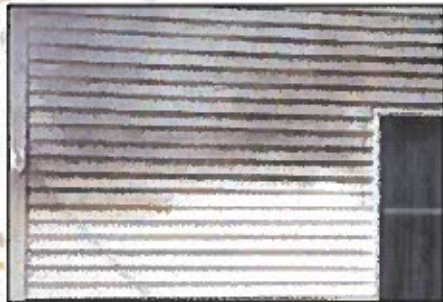
Mildew on painted exterior siding
