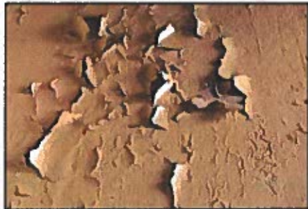
Peeling paint on interior wall
