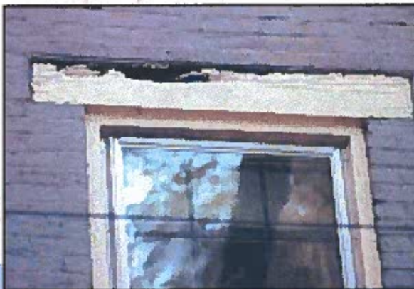
Rot caused by fungi feasting on wood window lintel.
