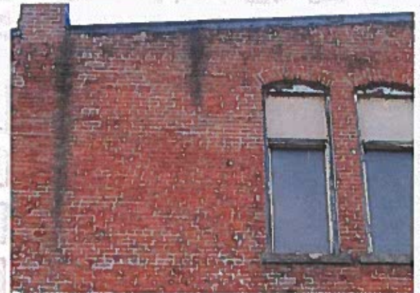
Dirt and stains on brick caused by runoff from the roof and corroded metal coping
