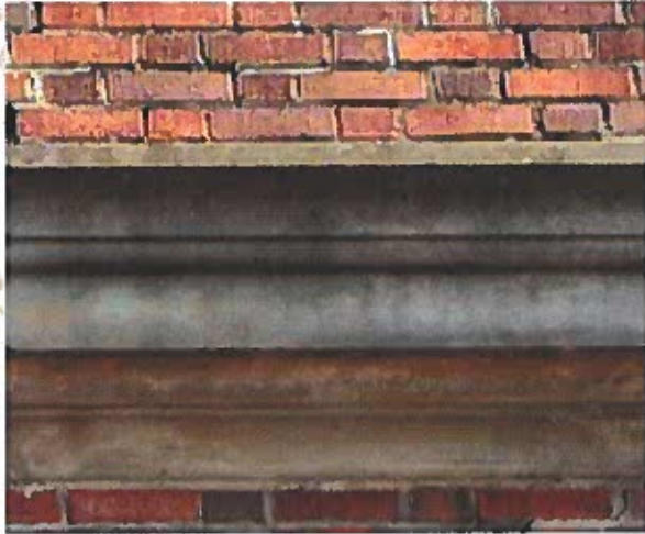
Disintegrating mortar and open mortar joints in masonry wall
