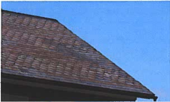
Good example of the appearance of a pattern on a historic roof.
