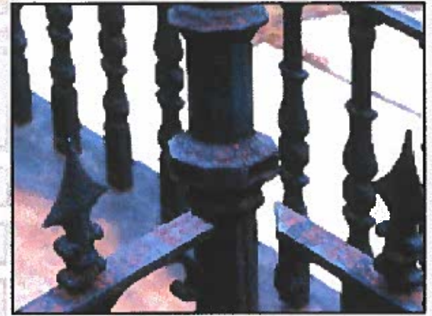
A corroded metal fence has failed at connections between the railings and the post.
