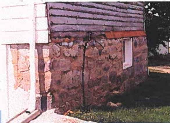
A foundation in poor condition.
