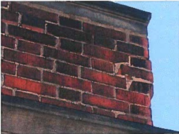
Displacement of brick by movement in the parapet wall
