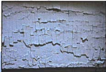
Alligatoring paint on exterior siding
