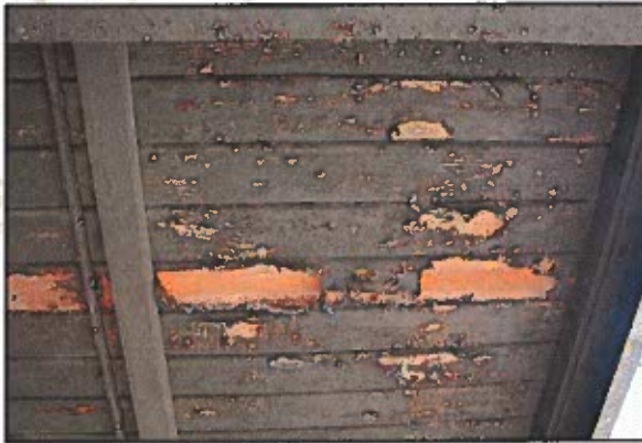
Paint failure on the underside of a wood canopy.
