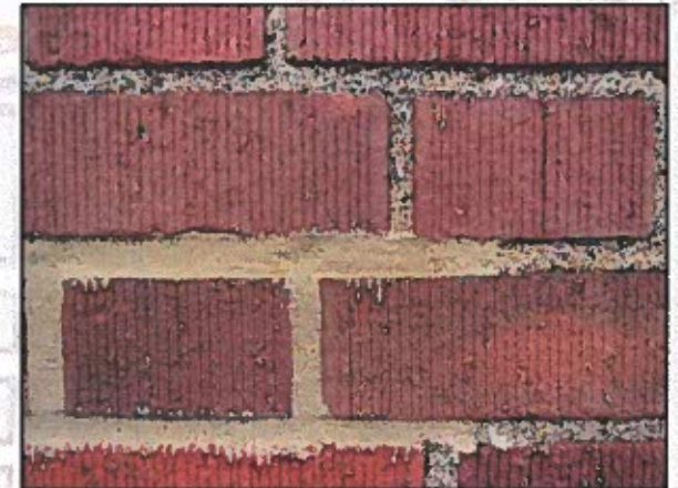
Recent poor repointing. New mortar is on face of brick and does not match original mortar in color, texture or tooling
