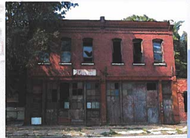
Lack of minimum maintenance over an extended period may render a building beyond rehabilitation.
