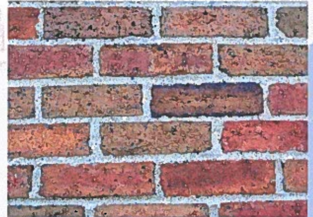
Damage to brick caused by sandblasting.
