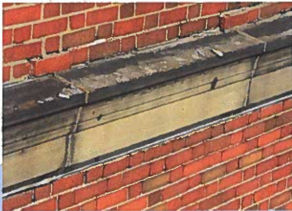
Loose brick falling out of wall due to poor conditions of mortar joints
