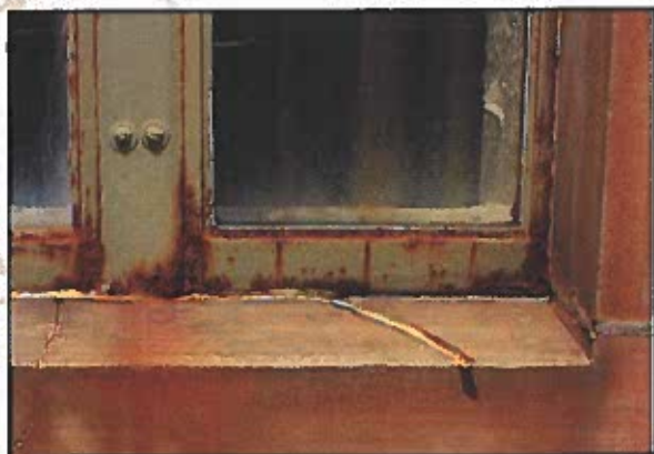
Corrosion/rust on a metal window sash resulting from exposure to moisture and air
